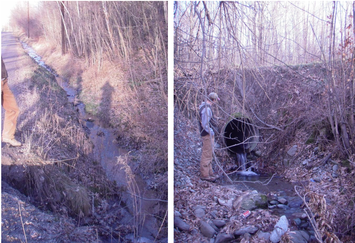
Figure 22. This culvert near 2982 Perley Rd. is too short, resulting in steep, erodible banks. Culvert inlet shown on left; Outlet is on the right.
