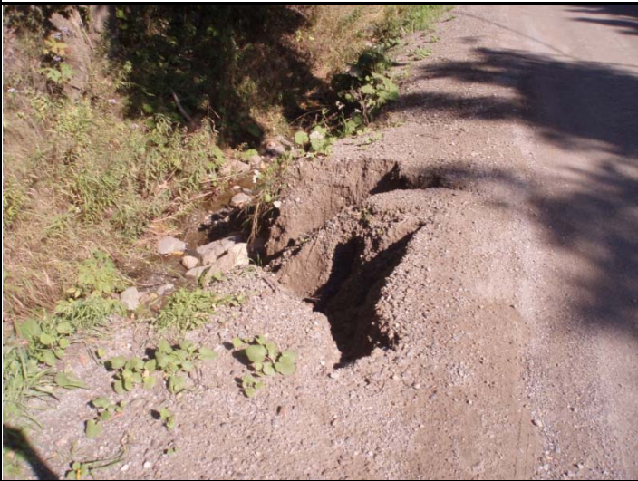
Photo 1. Road falling into ditch
