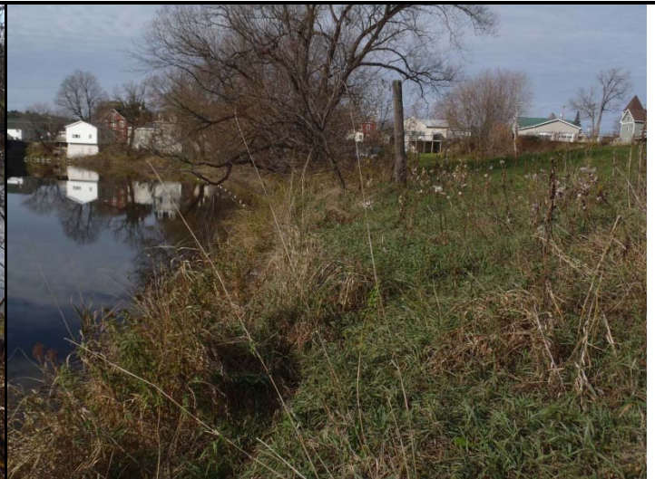
Photo 2. Bank erosion due to lack of vegetation
