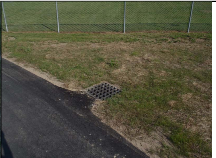
Photo 2. New catch basin at WW plant
