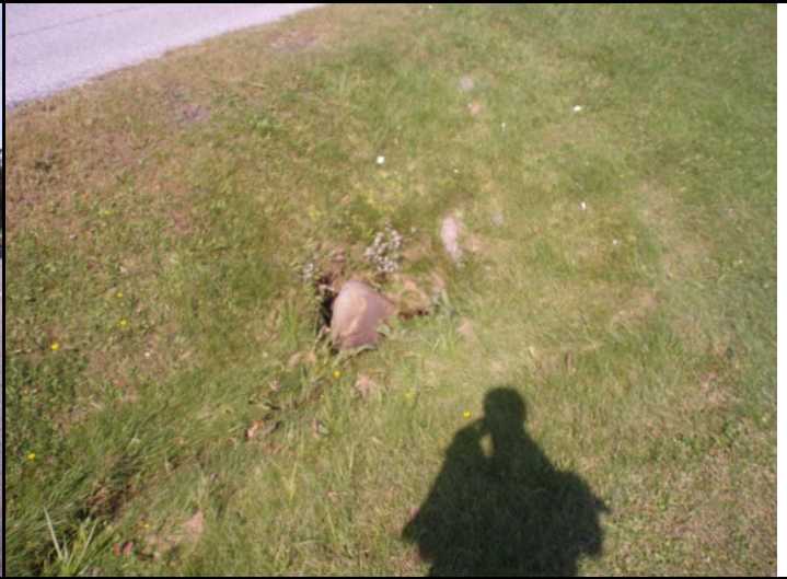
Photo 2. Ditch to undersized culvert
