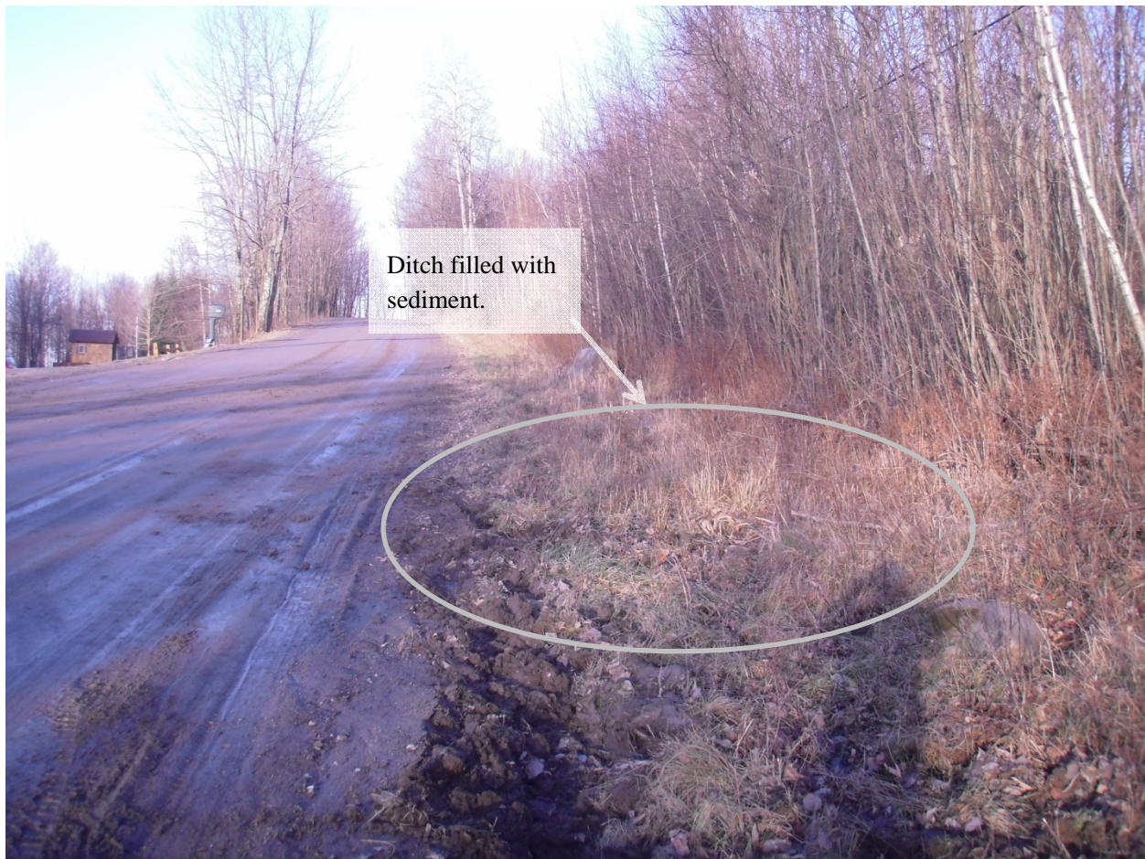
Figure 5. Ditch along Perley Road has become filled in. Diverted water is eroding the road surface.
