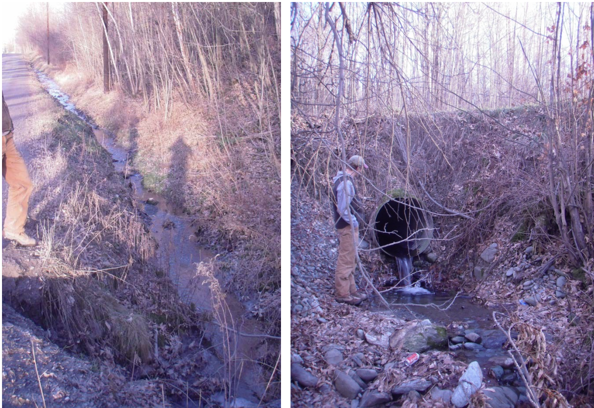
Figure 6. This culvert near 2982 Perley Rd. is too short, resulting in steep, erodible banks. Culvert inlet shown on left; Outlet is on the right.
