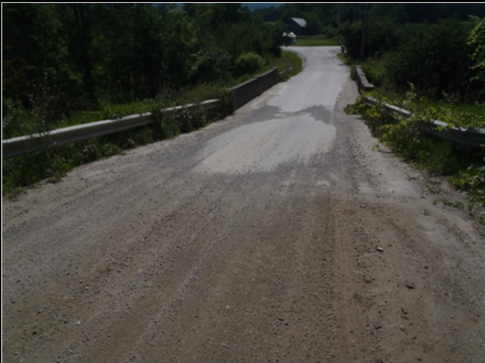
Photo 1. Sediment build up
