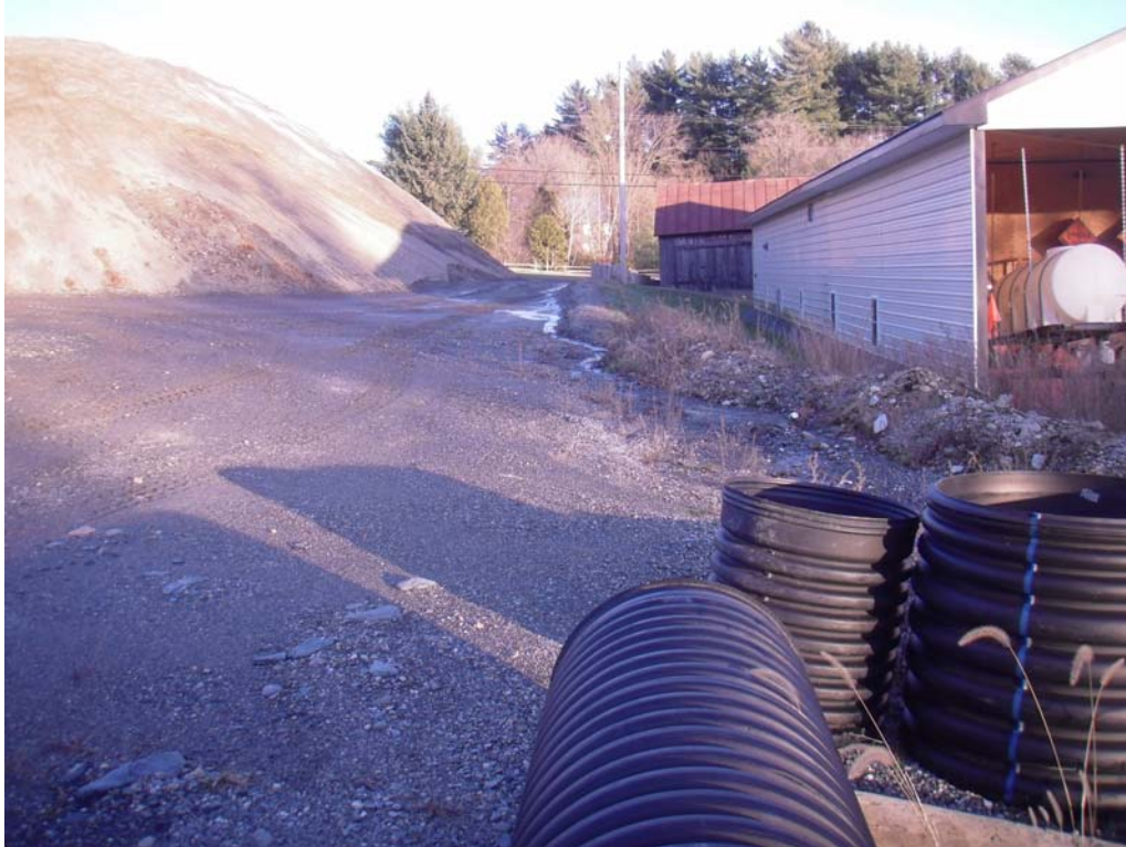
Figure 2. Material erodes from the stockpile and is carried offsite via the swale shown in center of photo.
