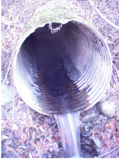
Figure 23. Corroded 36" culvert on Perley Road.
