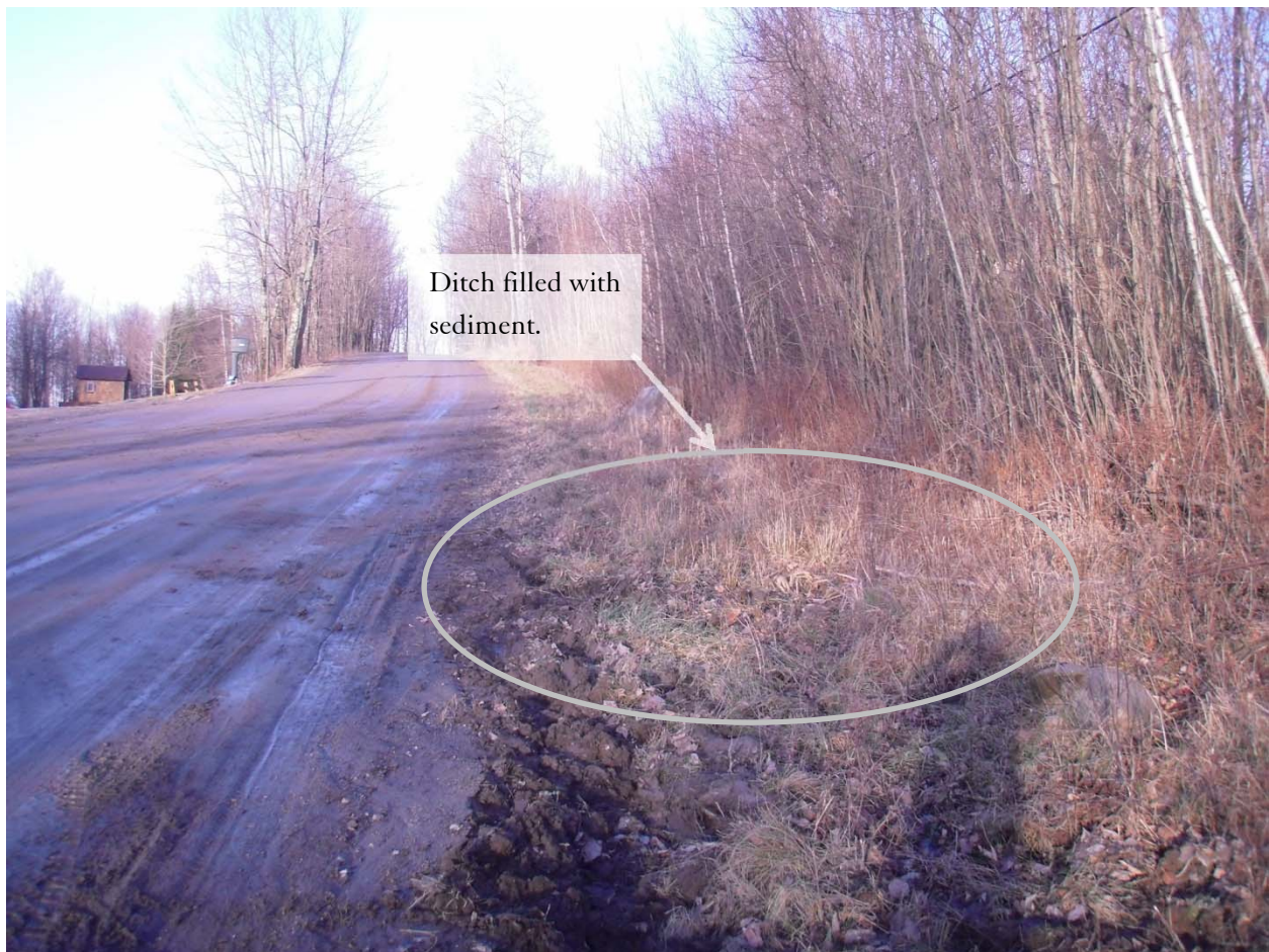
Figure 21. Ditch along Perley road has become filled in. Diverted water is eroding the road surface.
