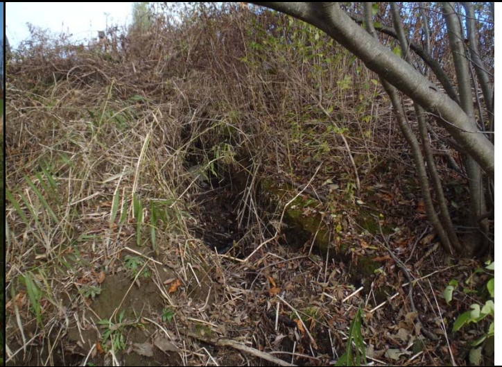
Photo 2. Ultimately causes 3 foot head cut (above)
